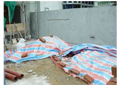
Figure 134 Covered stockpile with tarpaulin to minimise fugitive dust (Source: Environmental Protection Department)
