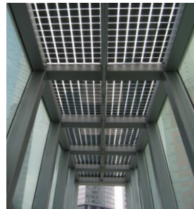
Figure 114 Photovoltaic installation in ZCB, Kowloon Bay
