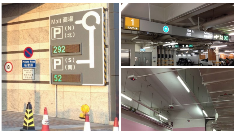
Figure 60 Parking guidance system (Source: Kai Shing Management Services Limited)
