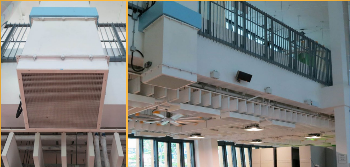
Figure 76 Windcatcher in ZCB (Source: ZCB, Construction Industry Council)
