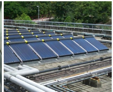
Figure 115 Solar hot water system
