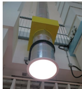
Figure 116 Light pipe in Zero Carbon Building (Source: ZCB, Construction Industry Council)
