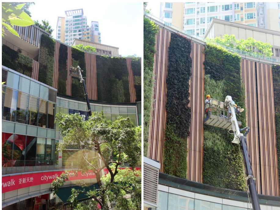
Figure 50 Maintenance of green wall façade in Citywalk, Tsuen Wan (Source: Sino Group)
