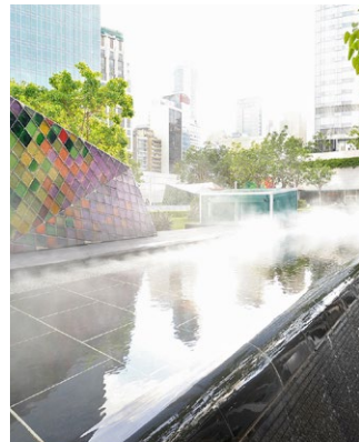
Figure 73 Water mist systems in ifc mall, Central
