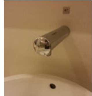
Figure 107 Water efficient fittings (Source: Kai Shing Management Services Limited)
