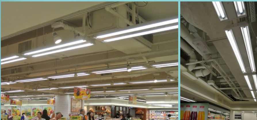
Figure 169 LED Lights, Wellcome at Causeway Bay
