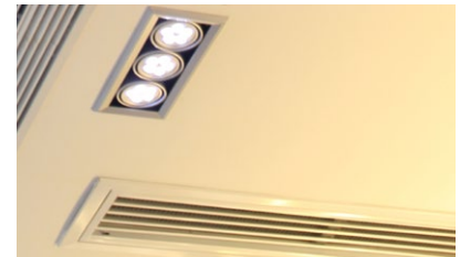
Figure 173 Use of LED lights
