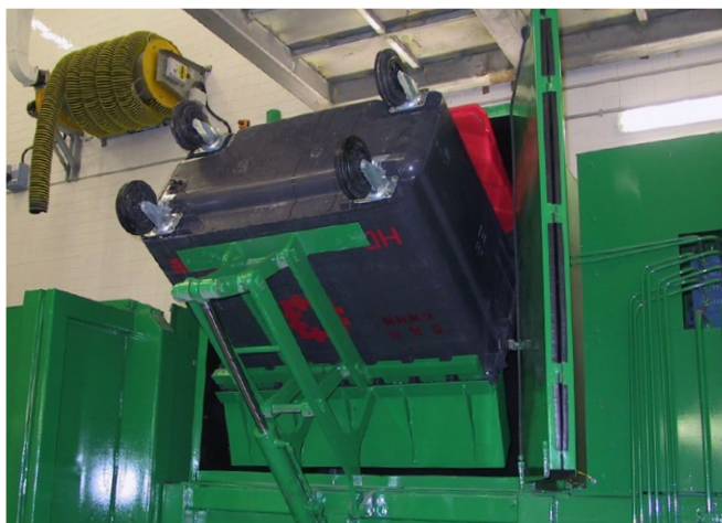
Figure 145 Central compactor system (Source: Hong Kong Housing Authority)
