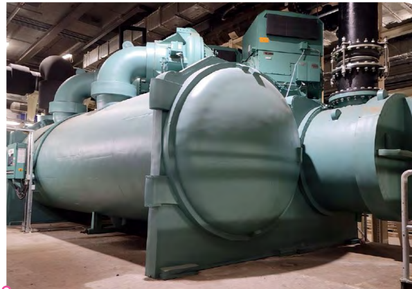
Newly replaced Variable-speed Chiller at Terminal 1 Chiller Plant
