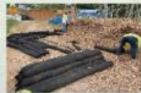
Filter media for treating surface runoff
